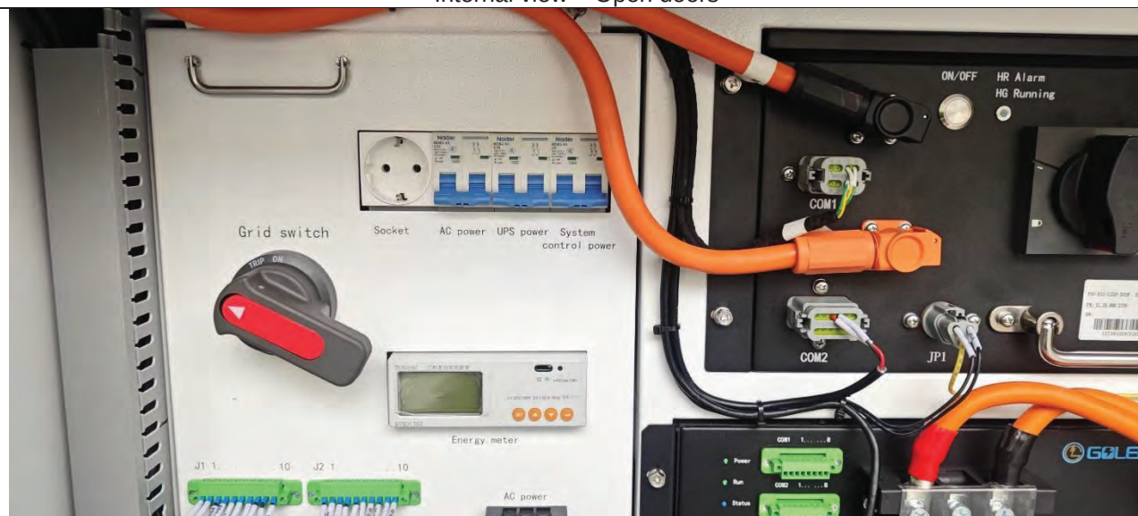
Overview view – Auxiliary, Circuit Breaker
